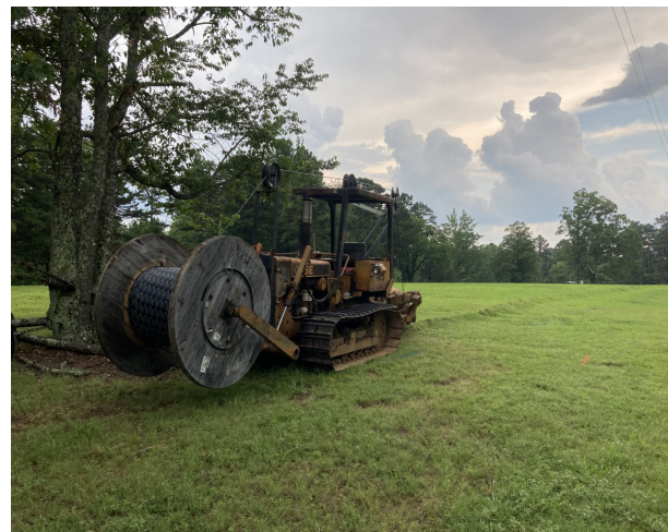
Large spools of internet cable await install at The Mount Eagle Retreat Center in Clinton, AR.
